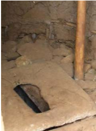
This latrine has a reinforced vent pipe that also serves as a support pole for easier use by PLWHA in a weakened state.
